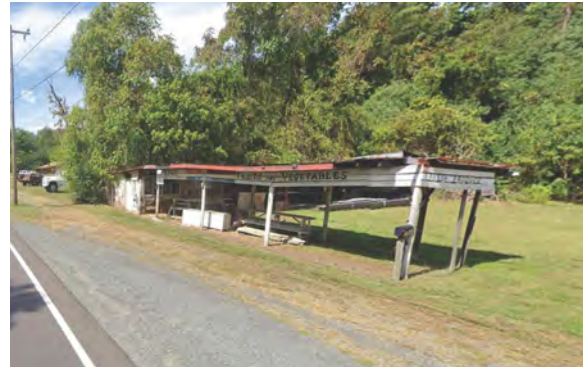
A Dilapidated Fruit Stand along U.S. Route 211 Source: Google Maps
